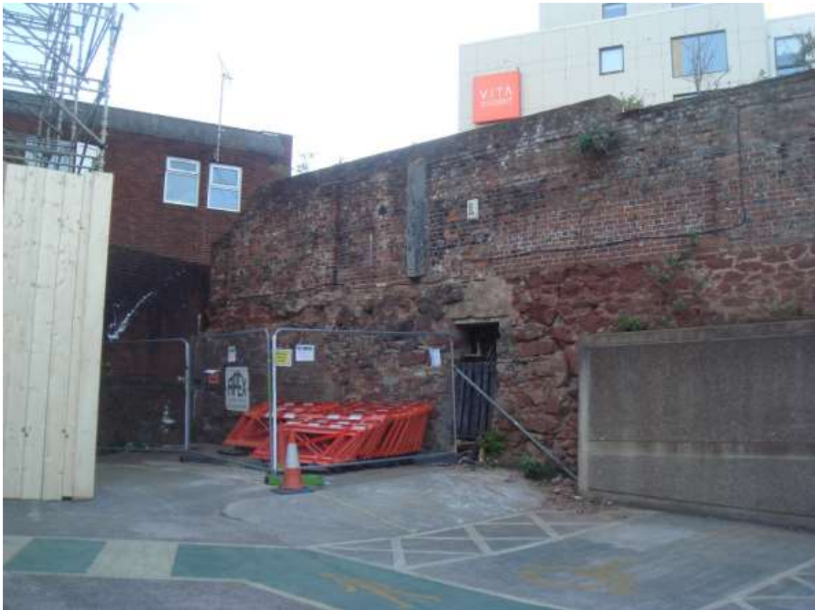
Photo 9: The surviving rear wall at 30-32 Longbrook Street where it meets the King Billy public house (partly obscured by a temporary scaffolding store at the time the photo was taken in June 2017). The lower courses of the wall in local Heavitree stone are believed to date from the 14 th or 15 th centuries. The upper storey of The King Billy public house (with its two adjacent windows) may be seen in the background.
